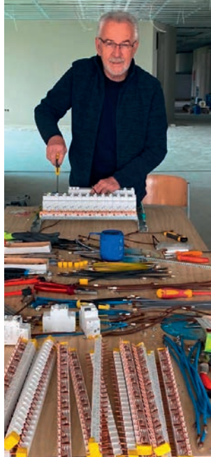
During the three-year construction period Bratko Horvat worked daily on the school construction site. The whole electrical system was installed using our own labor.
