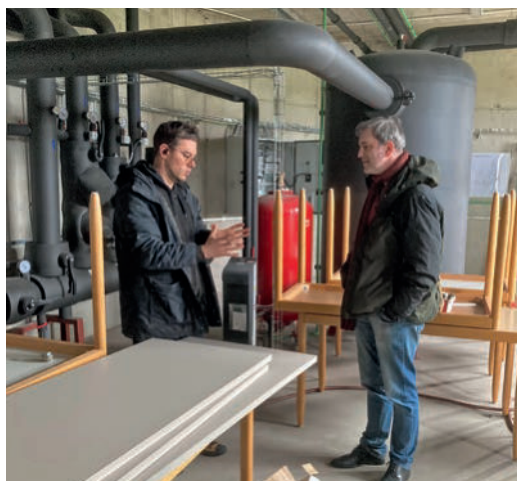
Petar Horvat (left) explains the heating pump in the new building, talking to pastor Thomas Ebinger.
